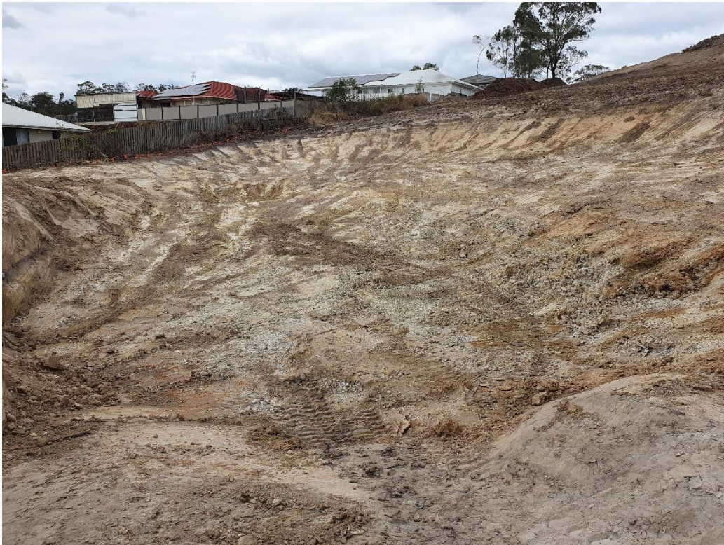
Stripping of a former dam to expose the natural soils prior to filling.
